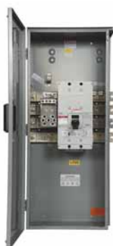
Main Circuit Breaker
