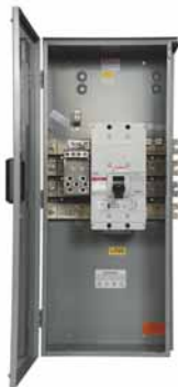
Main Circuit Breaker
