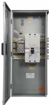
Main Circuit Breaker
