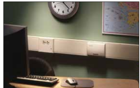
Ideal for offices and classrooms.
