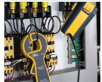
Inductive clamp allows you to induce a tracer signal on to the cable without affecting the low voltage signals on the circuit.
