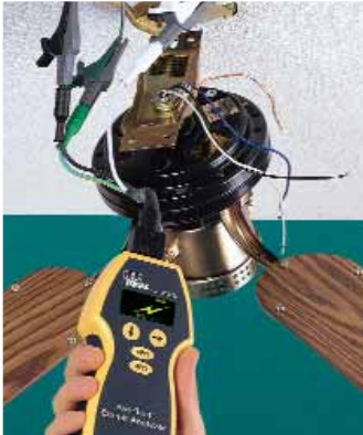
AFCI testing with alligator clips on an installed device.
