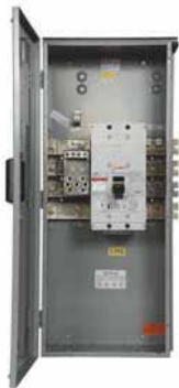
Main Circuit Breaker
