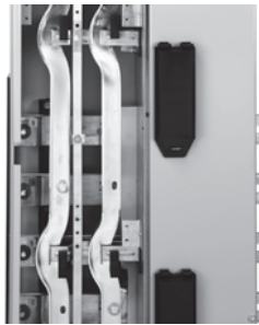
One-Piece Vertical Busbar
