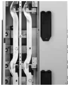
One-Piece Vertical Busbar
