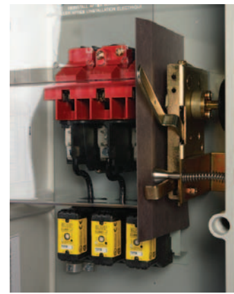
Enhanced Line Shield and Interlock Defeater
