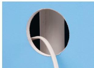
Pipe obstruction behind wall prevents the installation of a typical sconce box. Install mounting wing for 1/2" or 5/8" drywall. Pull cable...
