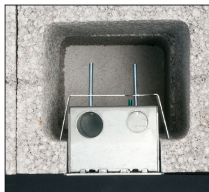
Insert the box in the opening in the block. (Top view shown)
