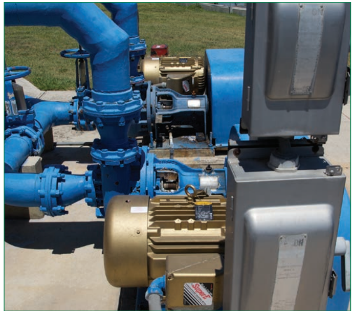
A Baldor Super-E motor and Inverter Control provide premium energy efficiency and improved process control to a municipal water treatment facility.
