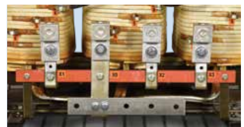
Expanded neutral bar for multiple customer connections
